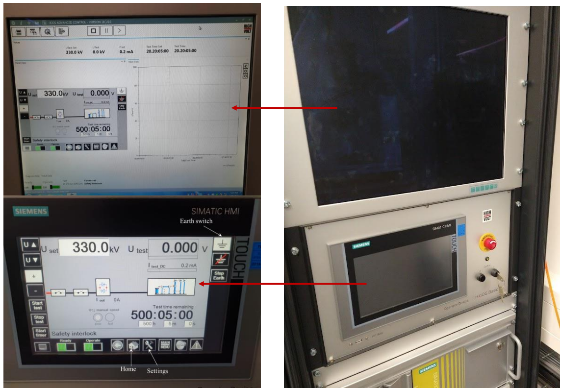
Figure 3.22 HiCOs computer-based software for controlling the DC generator.
